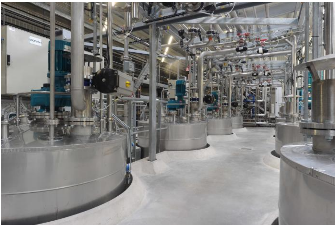
FuturoI™ pilot - Hydrolysis and fermentation workshop.
